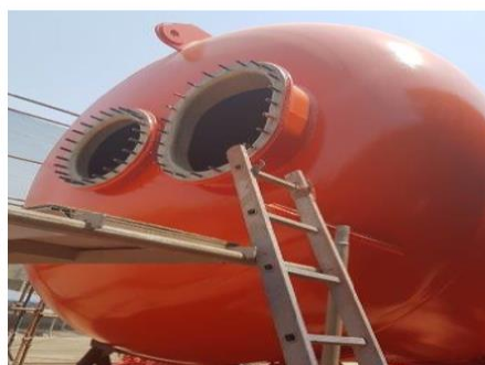
Figure (2) HCl Acid Tanks (prismatic and cylindrical types) during Fabrication Phase [Courtesy of OML (Overseas Marine Logistics L.L.C.)]
