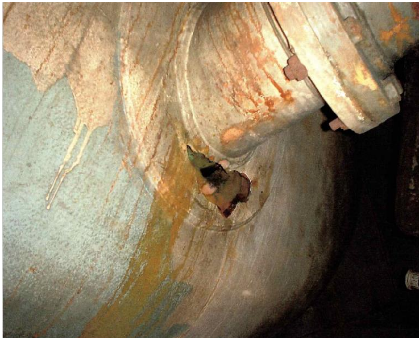
Figure (4) a hole resulting from severe corrosion due to HCl leakage from rubber coating in way of the suction nozzle of an acid tank [The photo was taken during the author experience with GL]
